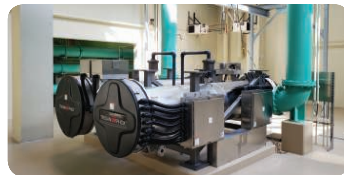
Barr provided engineering design and construction administration for the City of New Brighton's advanced oxidation process treatment system.
